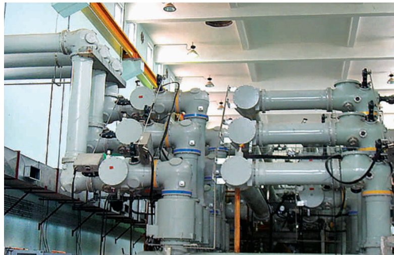
400 kV GIS Switchyard at North Chennai TPS
