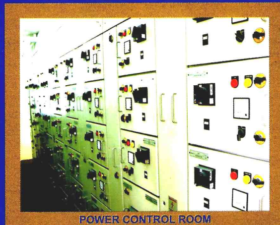
POWER CONTROL ROOM
