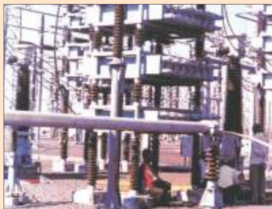
400 kV series Capacitor Bank for POWERGRID, FSC Wardha
