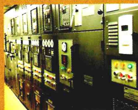
VFD CONTROL HOUSE
