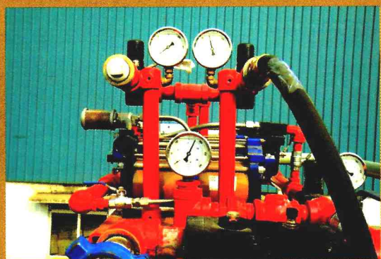
PRESSURE MONITORING SYSTEM
