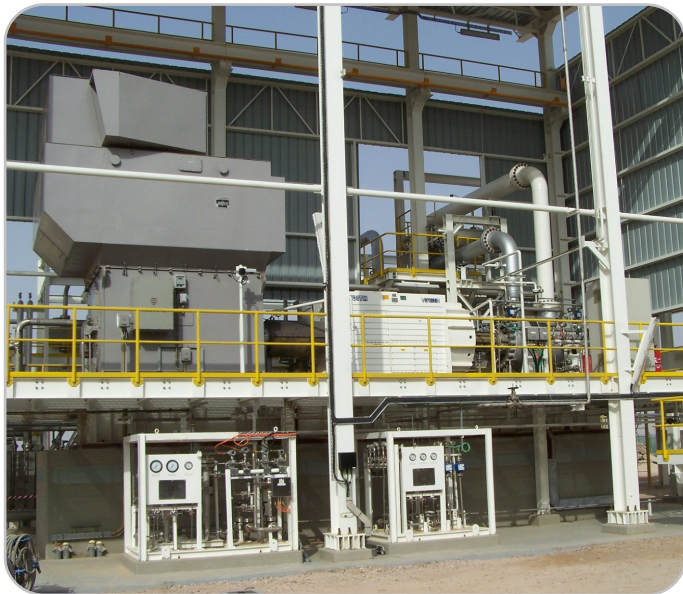
Depletion Compressor installed at Oman
