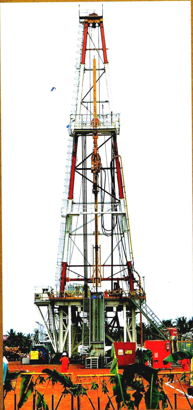
FIRST AC VFD RIG COMMISSIONED AT ONGC RAJAHMUNDRY
