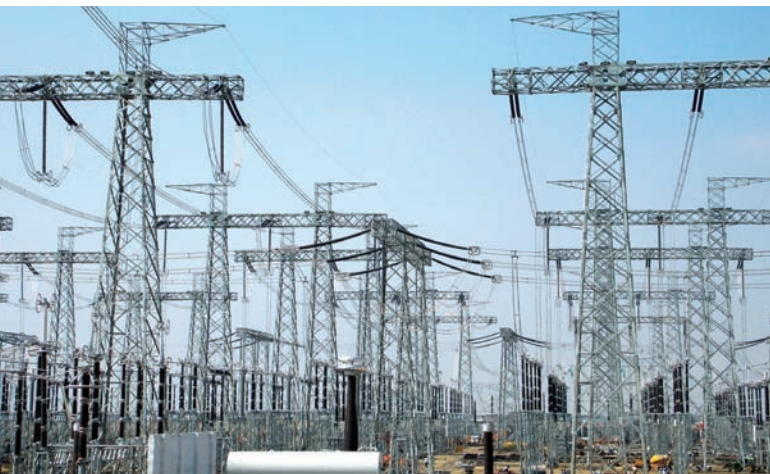
765 kV Substation at Raichur
