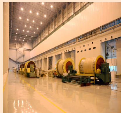
Air Conditioned Transformer Winding Mfg. Bay
