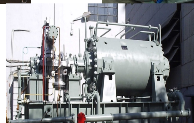
Steam turbine driven H2 Recycle Compressor for motor spirit quality upgradation
